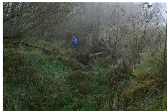
Figure 1. A naturally occurring high-flow side channel augmented with large wood structures in Salmon Creek (photo by GRRCD).
