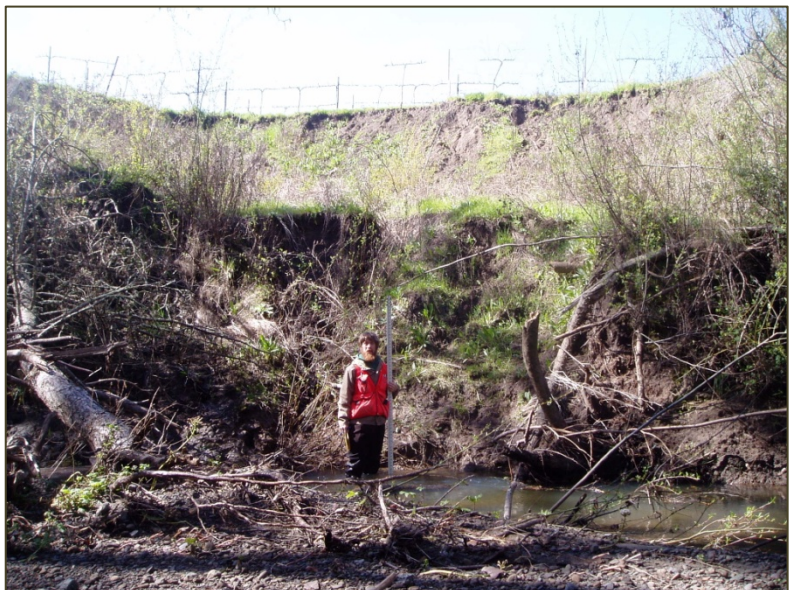
Bank Collapse/Erosion. Photo courtesy of Matt O'Connor.
