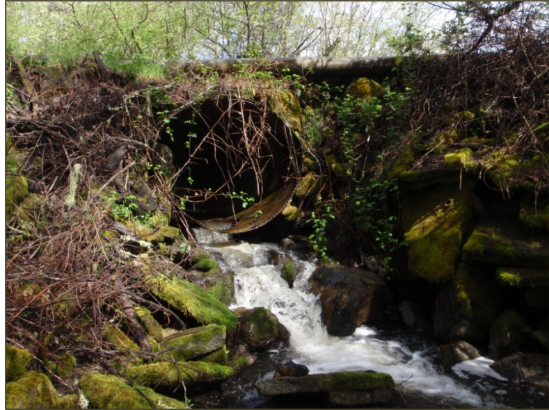
Stream crossing in poor condition on upper Green Valley Creek. This crossing is a barrier to coho salmon passage.
