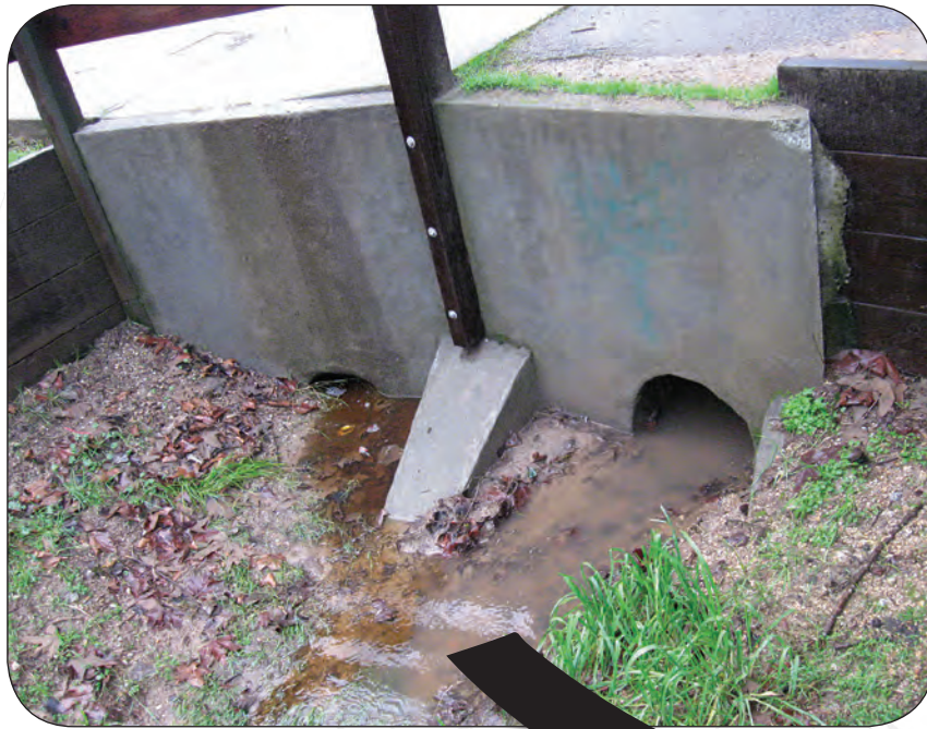
RUNOFF FROM THE SURROUNDING HOMES AND STREETS FLOWS THROUGH THIS STORM DRAIN...
