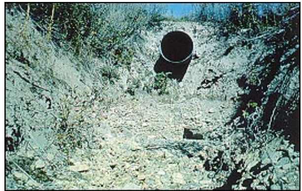
A culvert not installed at the existing stream gradient can degrade the channel.
